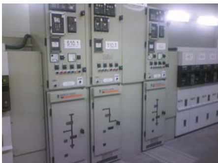
One of the existing Switchboards to be monitored by the NCS
